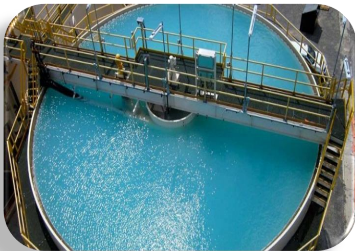
Lahore Water and Wastewater Management Project Pakistan USD505,000
